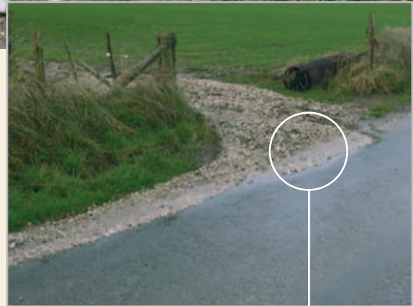
Runoff onto adjacent road
